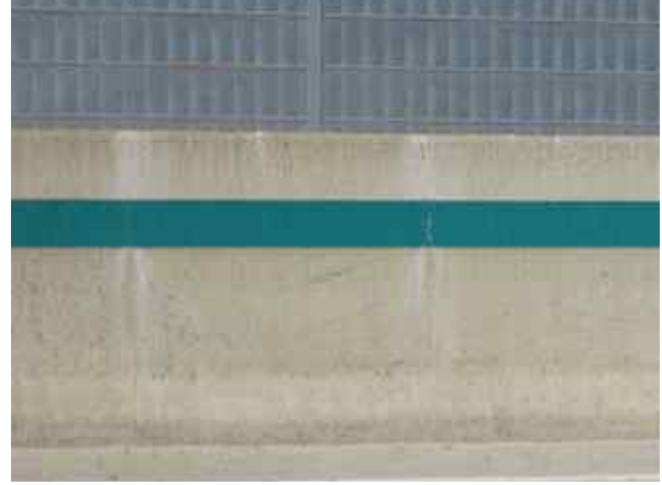
S3 방호벽 균열(0.2mm/1.5m)
